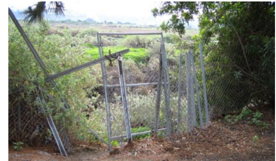
Broken fence at area A
