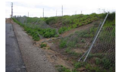
Fallen fence at area C
